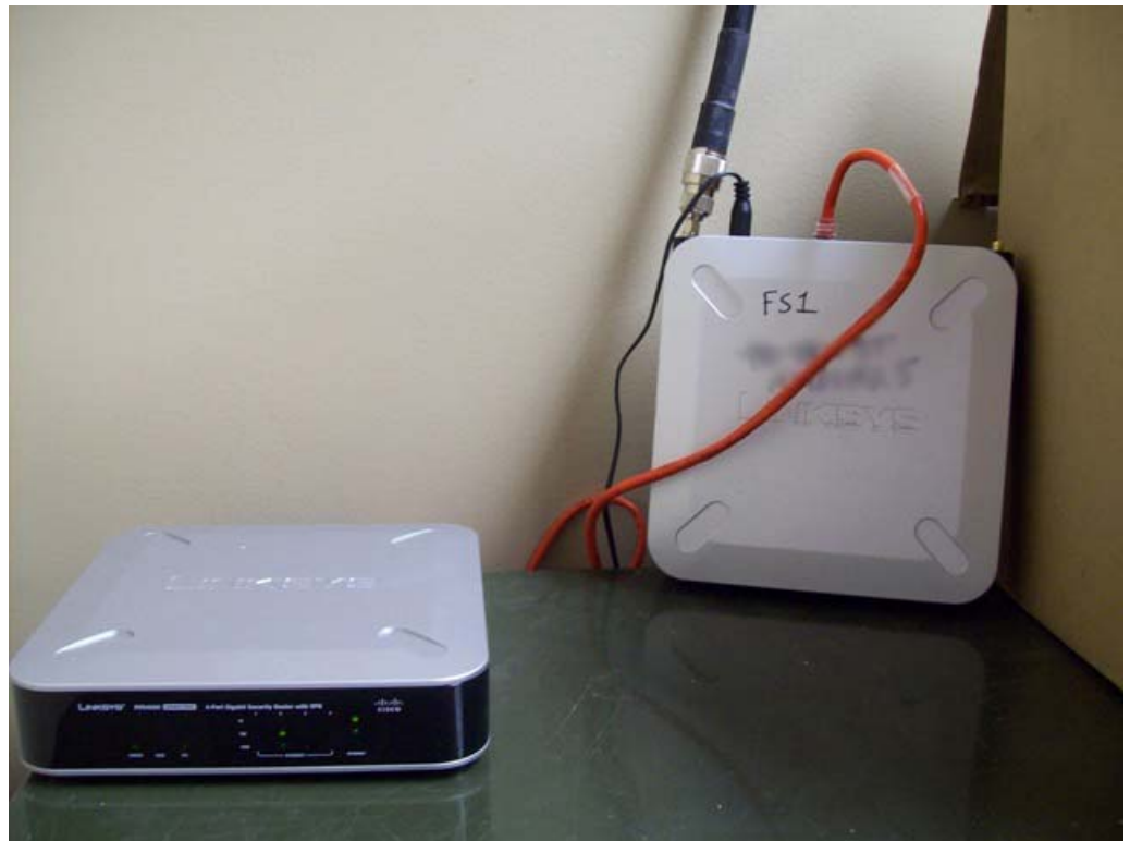
The Fire Department's WAP200 is connected to the LAN through a Linksys Business Class router.
