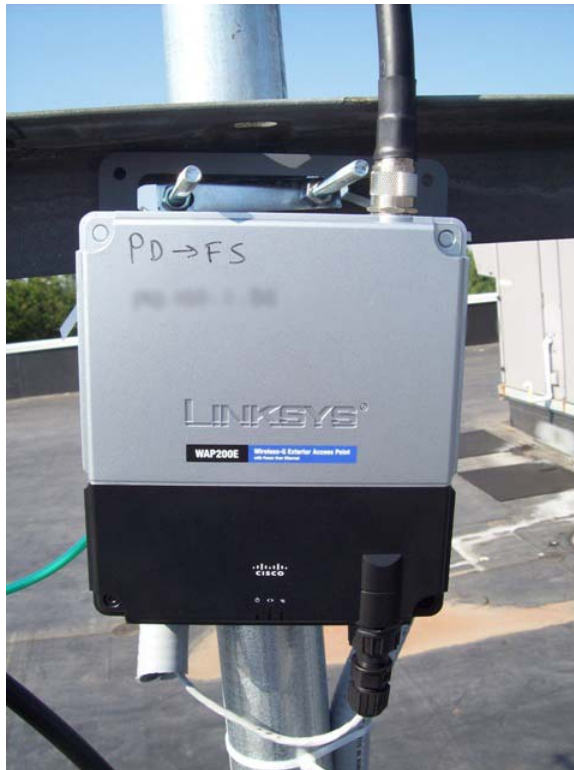
The WAP200E is mounted on the Yagi antennae. Note the antenna cable on top, network cable on bottom, and an unseen grounding wire attached to the back. The antenna is also grounded. Both ground wires are attached to the grounded antenna mount.
