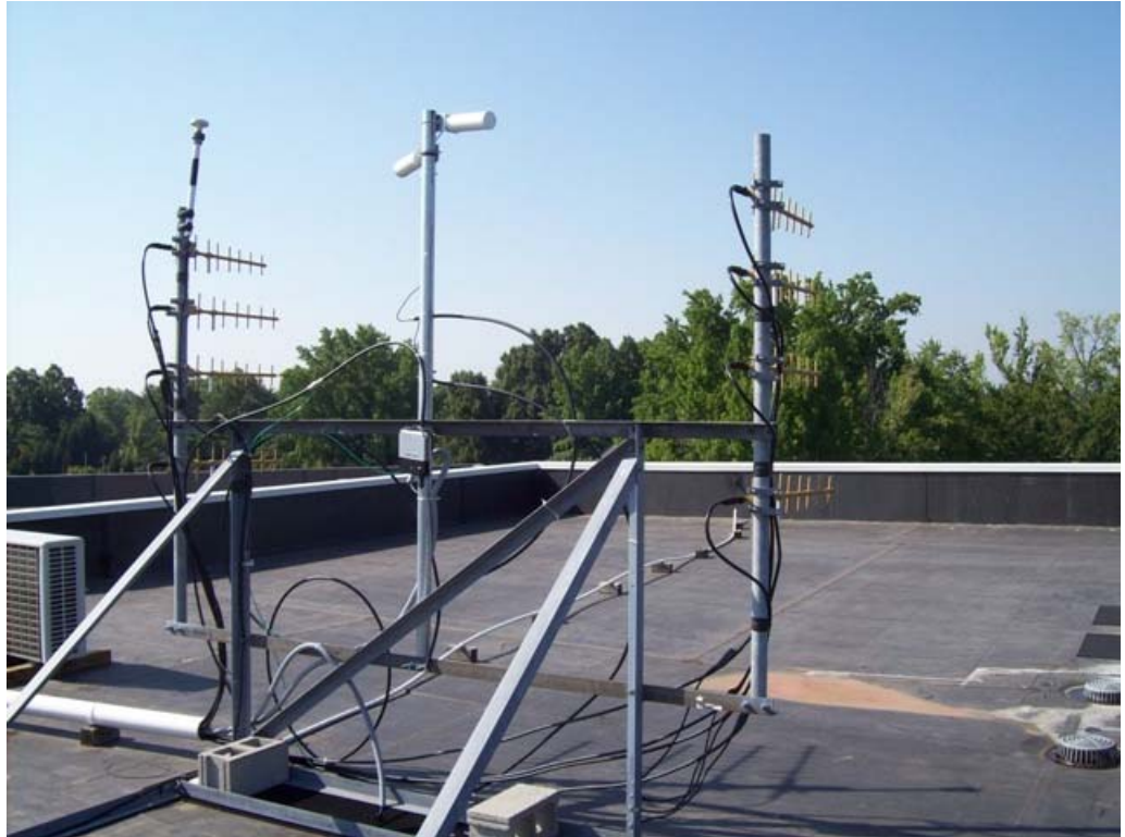
The antenna station provided an excellent foundation for mounting the WAP200E and Yagi antennae.
